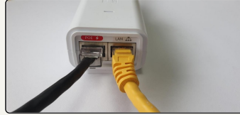
Black antenna cable in POE , yellow ethernet in LAN .
